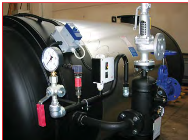
Figure 4 Safety and control instruments on an horizontal UNI-MATIC UM steam generator.
